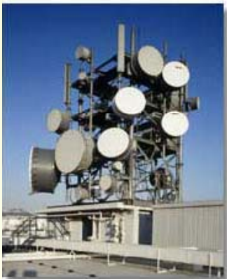
Typical Mobile Telephone Site on building.
