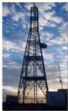
Typical Mobile Telephone Site on the ground
